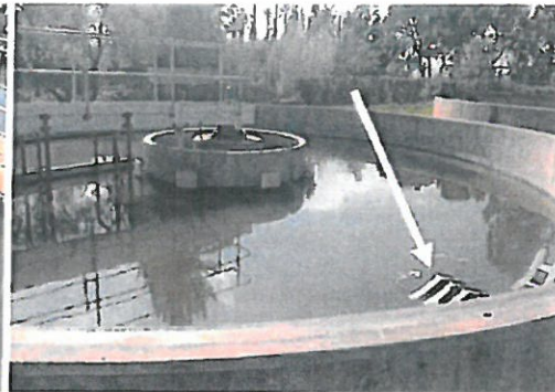
Fig10: Settling tank (material floating)
