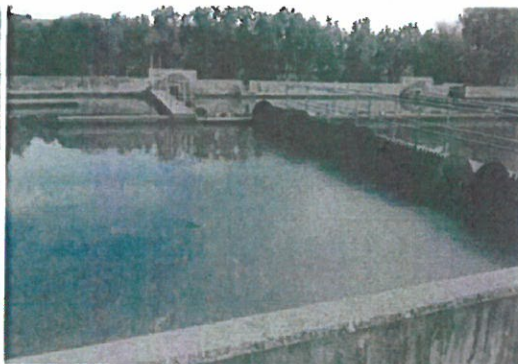
Fig4: Aerator not functional
